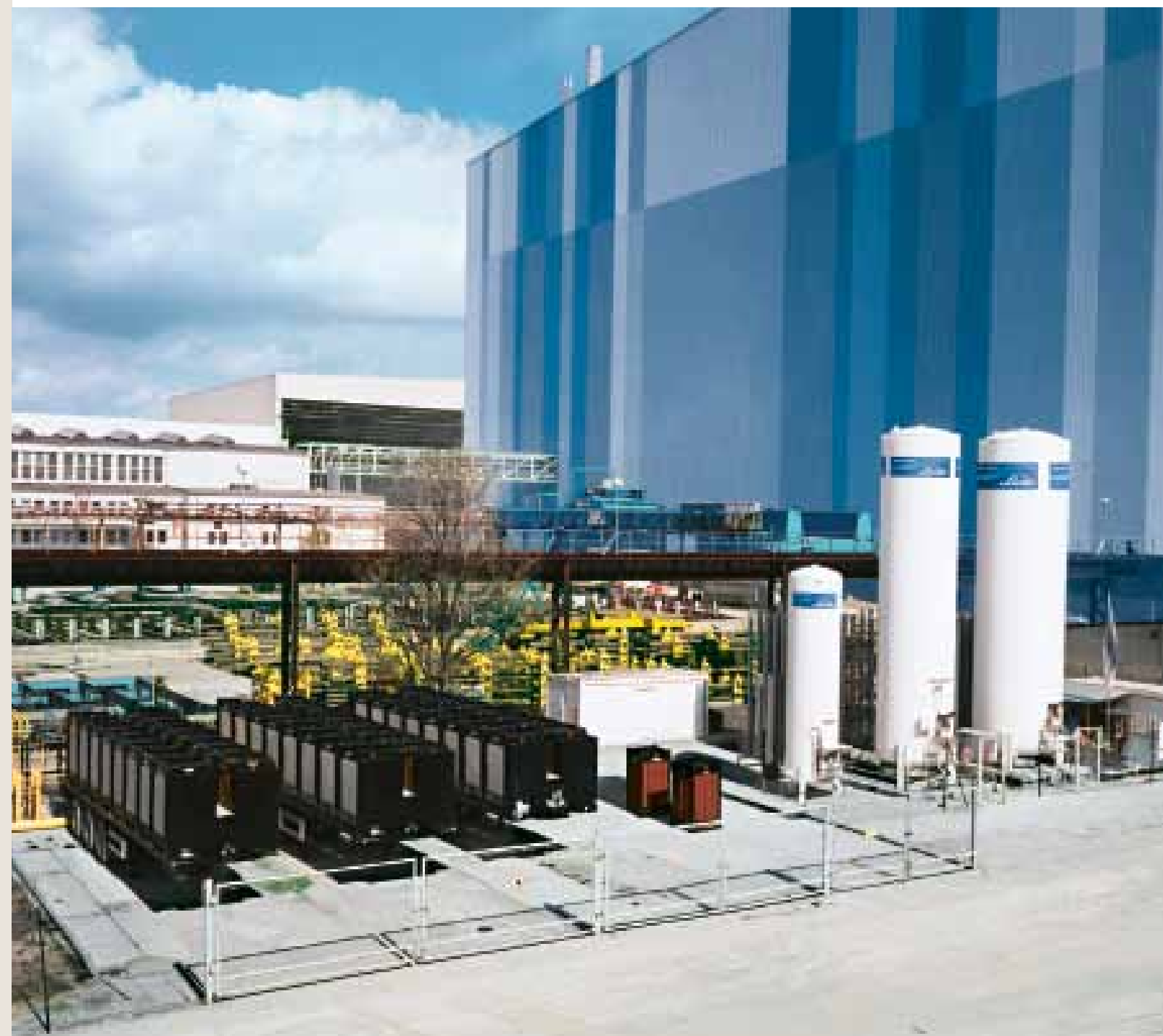
Gas supply point: three trailers for acetylene and liquid tanks for argon, carbon dioxide and oxygen.
