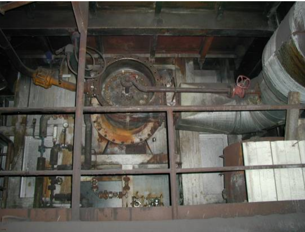
4 MW air-fuel installed, before REBOX ®
