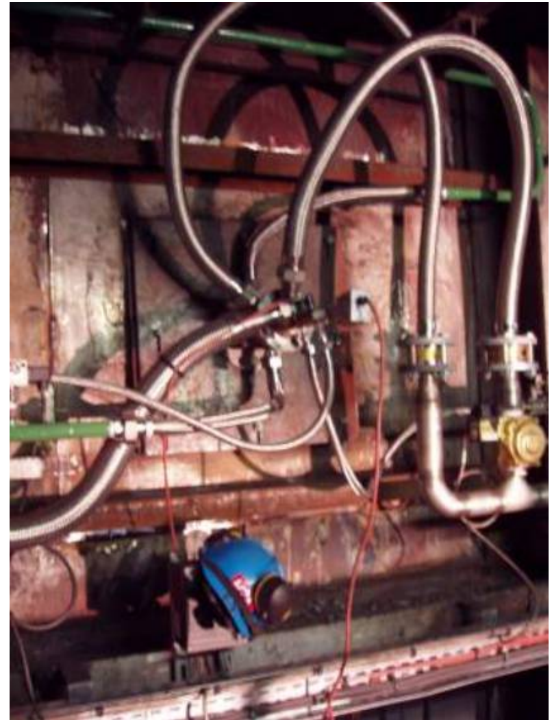
2.5 MW Flameless Oxyfuel Installed 15
