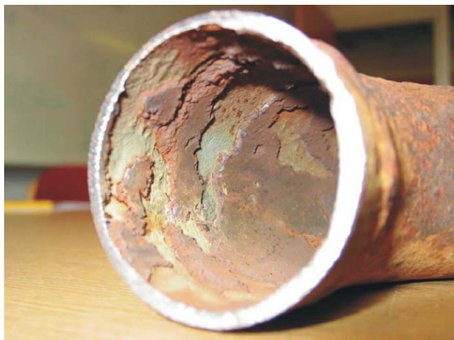
Figure 2: Pipe corrosion caused by carbonic acid
