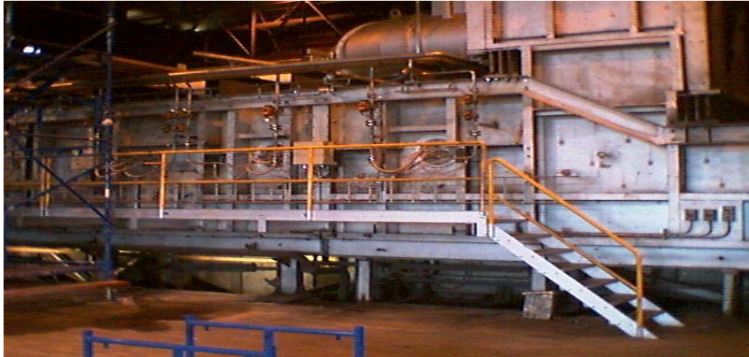
Figure 2. The photograph shows a walking beam furnace in Sweden that has been converted to all oxyfuel operation using 26 flameless oxyfuel burners.
